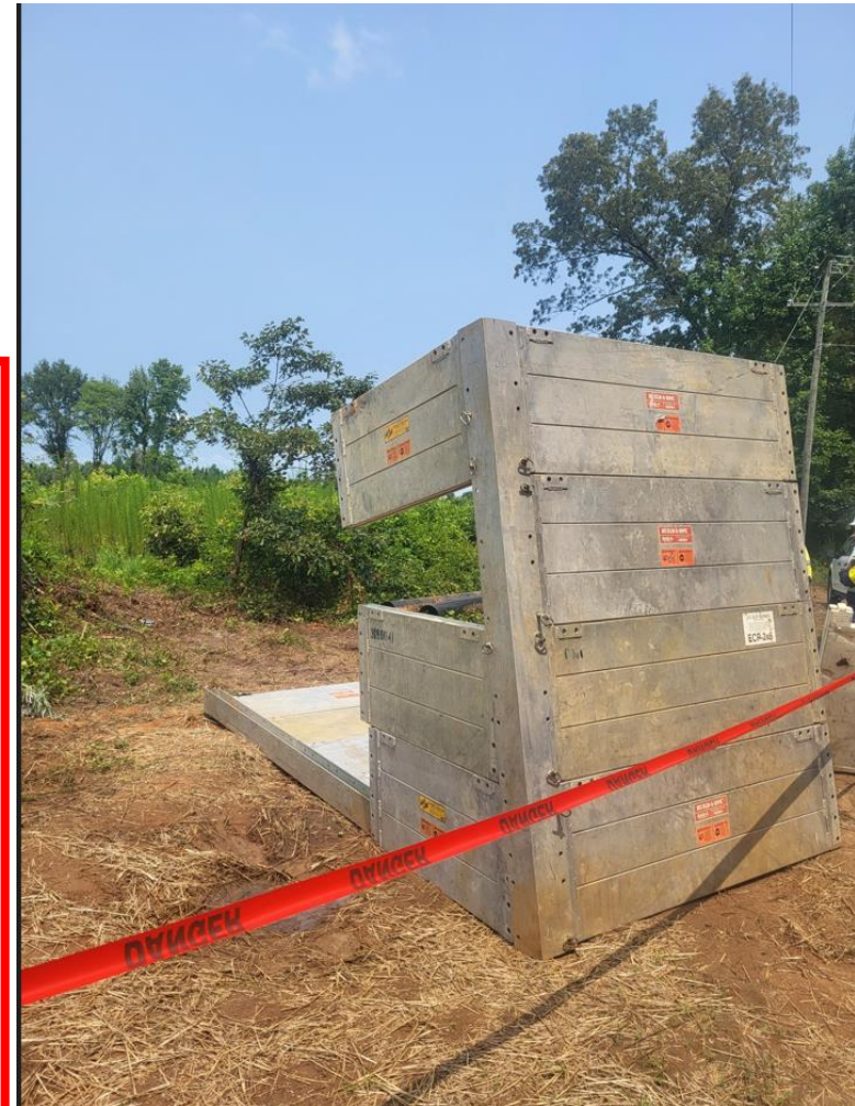
Accident scene showing modular trench box being disassembled.
