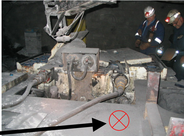
Employee's approximate location while disconnecting energized battery charging plug
